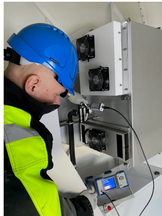
Figure 13 Calibrating a WRS400 X-band weather radar with a thermal power sensor during annual system calibration. Working space inside the radome is convenient for carrying out the test procedures.
